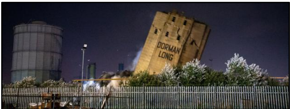
Figure 24 The Dorman Long tower mid-fall during its demolition in September, 2021. The Northern Echo . Available at: https://www.thenorthernecho.co.uk/news/19593244.report-reveals-cost-repairing-dorman-long-tower/
