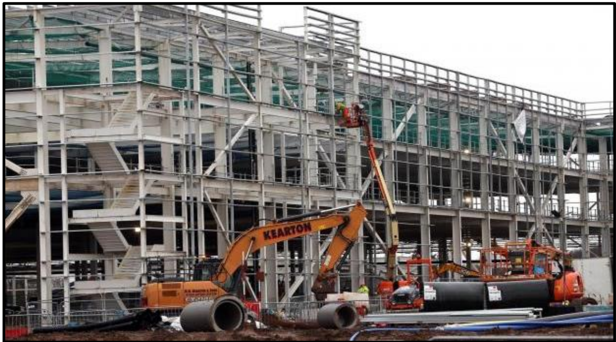
Figure 45 The Amazon site while under construction at Symmetry Park. (Sarah Caldecott © [2020]). Available at: https://www.thenorthernecho.co.uk/news/18440030.amazons-first-fulfilment-centre-north-east-officially-opens-darlington/
