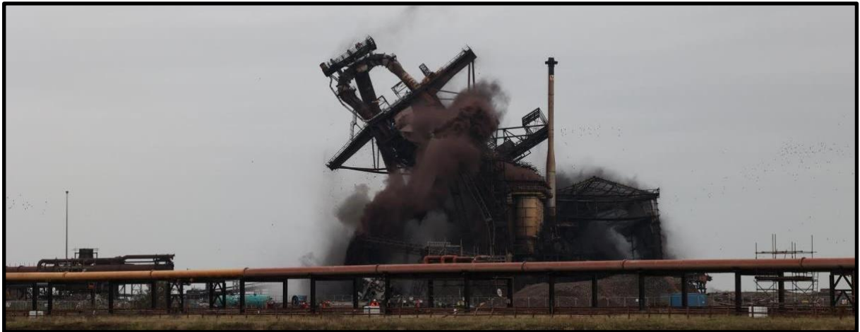
Figure 23 Teesside skyline being permanently altered as the SSI steelworks furnace at Redcar is brought down using 175kg of explosives. The Northern Echo . Available at: https://www.thenorthernecho.co.uk/news/23143694.redcar-blast-furnace-demolition-pictures-skyline-changes-ever/
