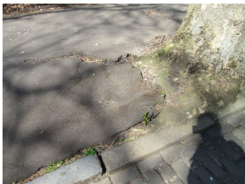
Image 4. Uneven pavement because of tree roots
